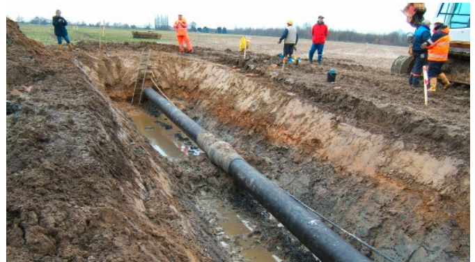
Excavation of metal loss defect and coating defect
